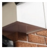
Over Fascia Ventilation
